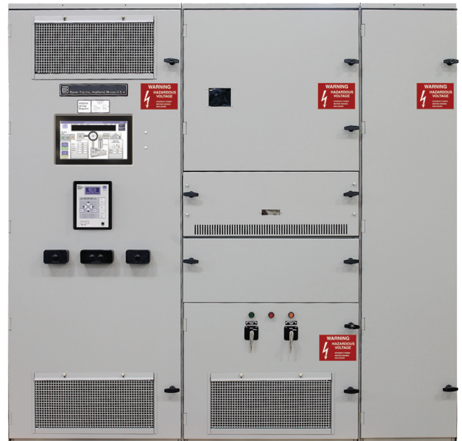
Figure 1 - IDP-1500: DECS-2100 Installation
