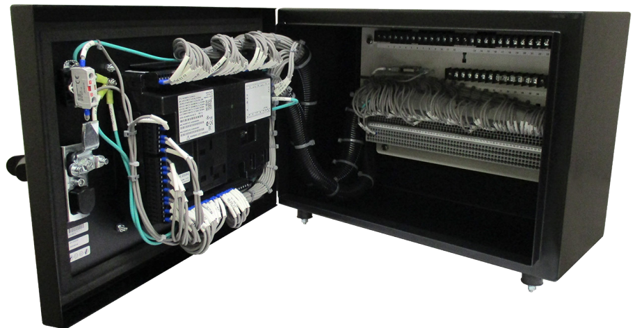
Figure 1 - Genset Top Mount Enclosure (door open)
