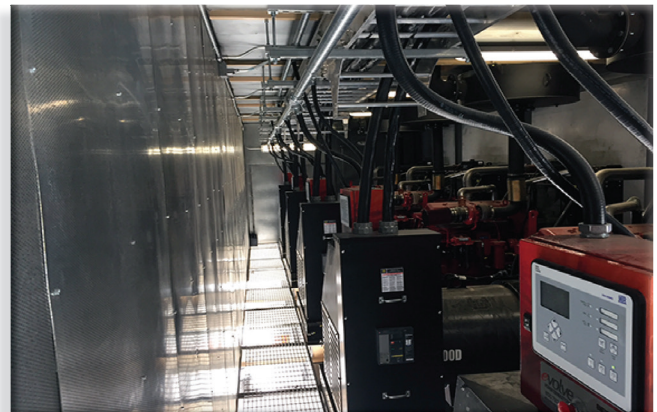
Figure 1 - Inside look at one of the two 5 generator systems
